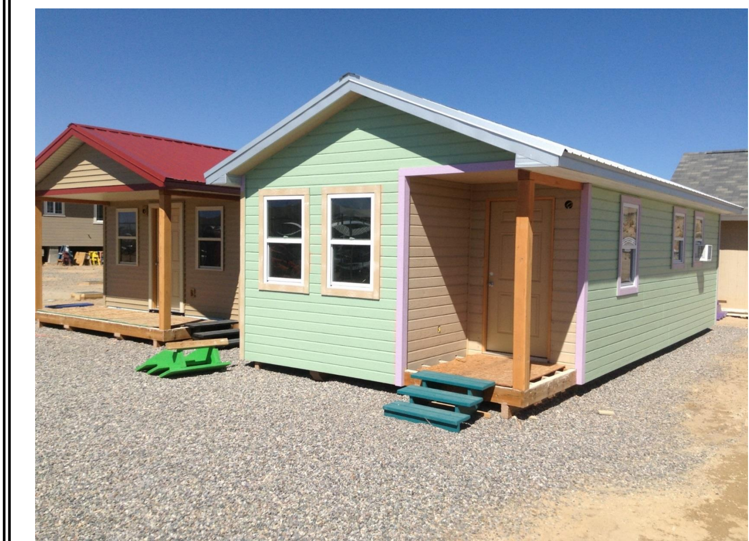
Fig. 3. Architectural plans and framing of house on SJC campus by Building Trades Program
